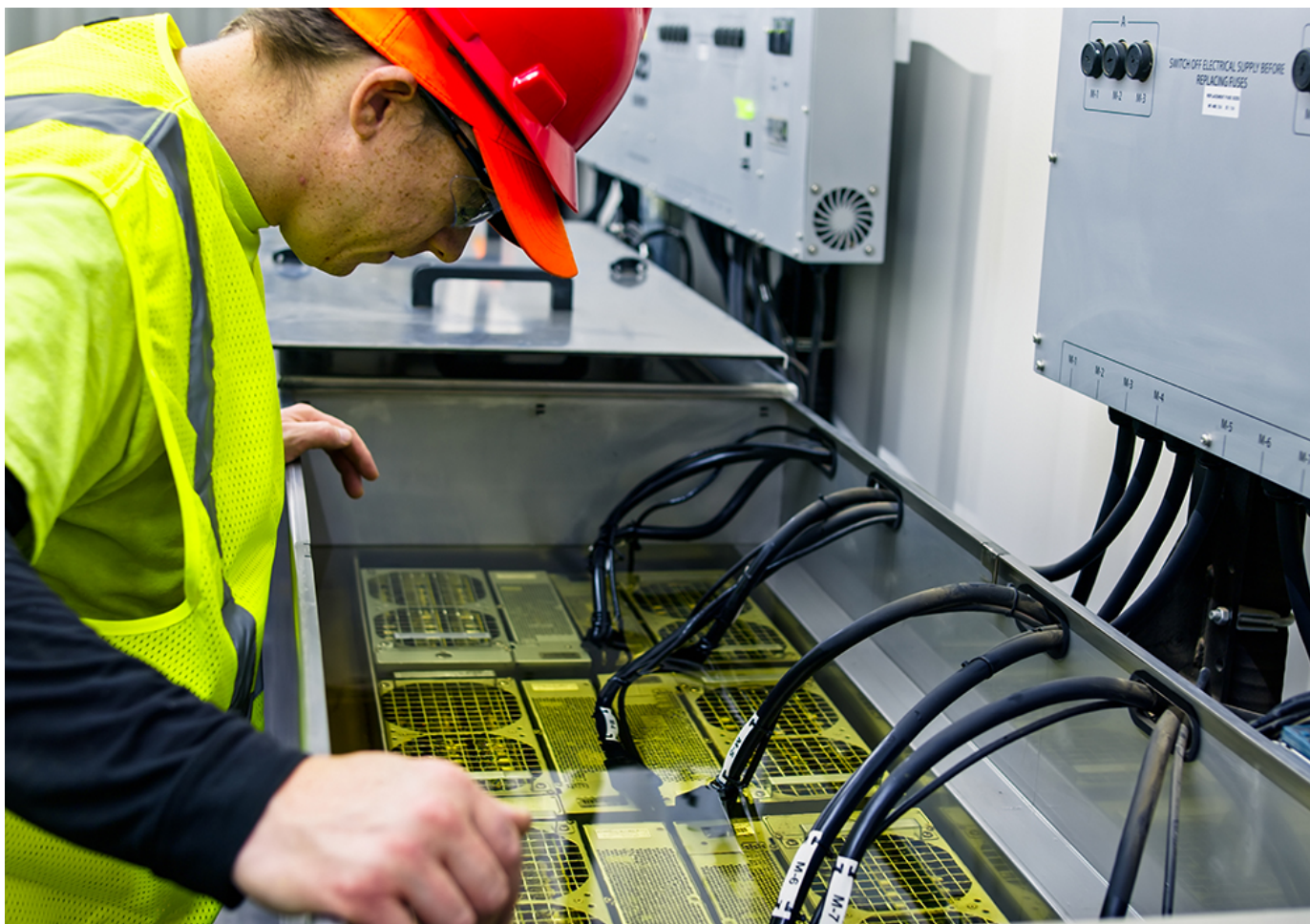
A North Dakota data center using nonconductive fluid to cool servers rather than air or water cooling systems (Credit: halbergman/E+)
